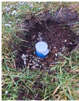
Figure 2. Installed dip well
